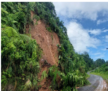
Figure 13c: Landslip at Qiolevu Road on 26 th . Source: Fiji Roads Authority.
